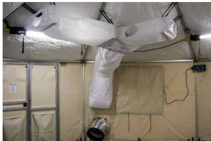
Plenum installed in SH-20 shelter
