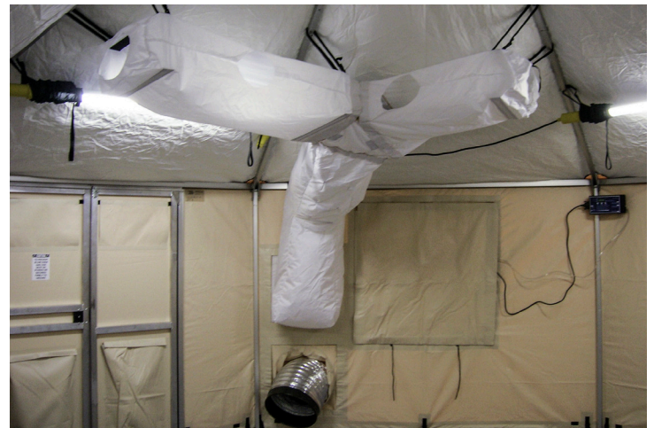
Plenum installed in SH-20 shelter
